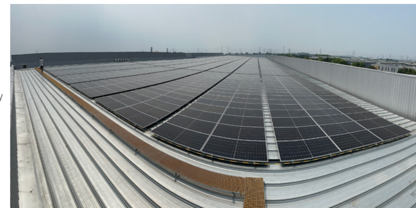
2MWH PV rooftop
