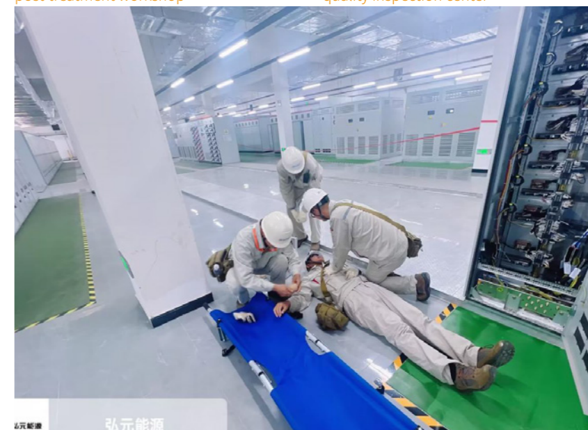
Emergency drill for anti-electric shock in electrical workshop
